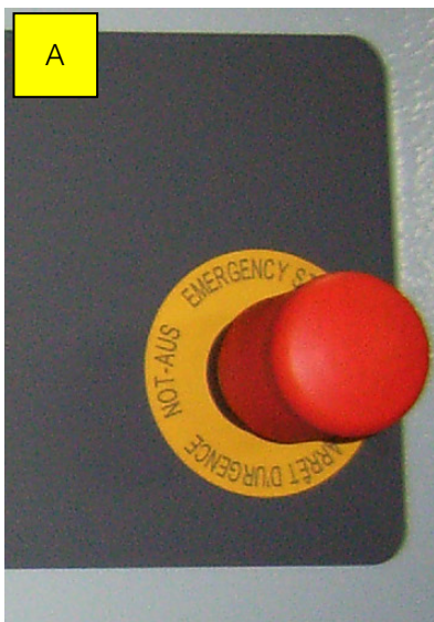
A EMERGENCY STOP at Communication Desk
